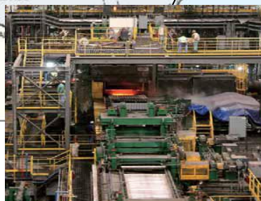
Jointly developed "Strip Caster (Castrip)" Technology with BlueScope Steel & Nucor Corporation (USA)
